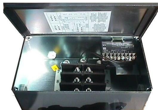
IP 54 Electrical box
